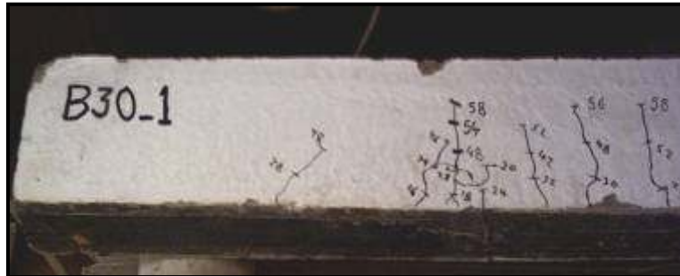
Figure (4.2) Crack pattern for strengthened beam B30-1
